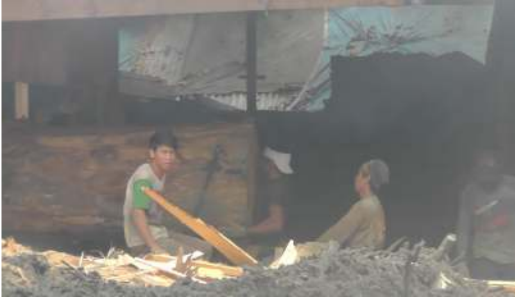
Figure 36. Workers without health and safety equipment
